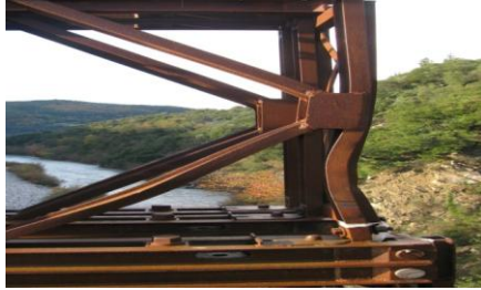
Photo 3. Corrosion of steel
