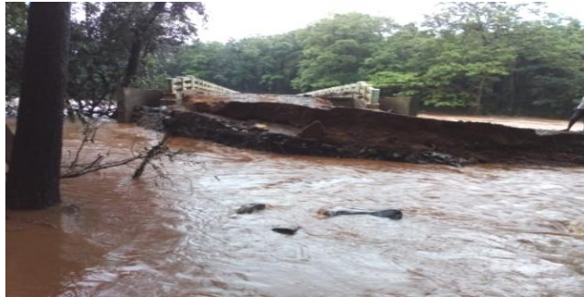
Photo 1. The approach is washed out
