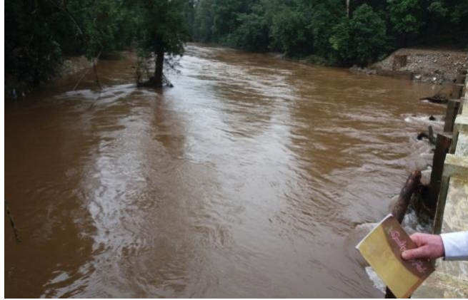
Photo 4. Vents choked up due to floating debris (trees) on U/s of the bridge
