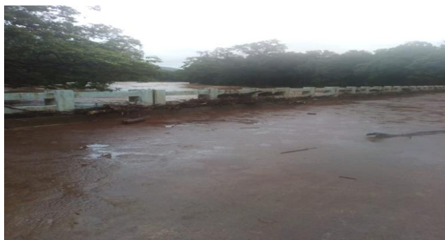
Photo 3. Water flowing above the deck. Even the openings of the R.C.C handrails are choked up with debris
