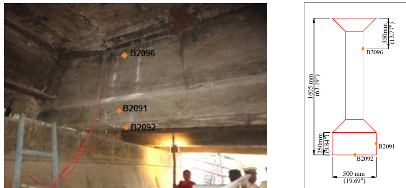
Figure 4(a,b). Position of gauges in the longitudinal girder near the abutment (Photometric view)
