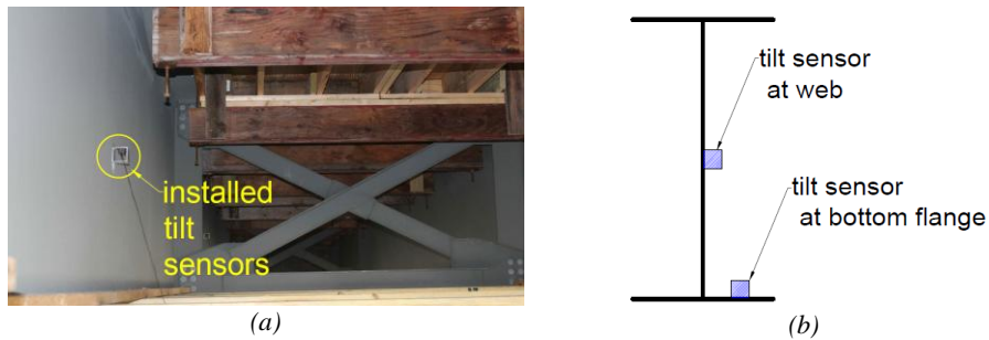
Figure 5. Installed tilt sensor in the bridge: (a) tilt sensor, (b) locations of tilt sensors
