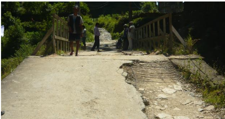
Figure 5. Concrete spalling in approach slab
